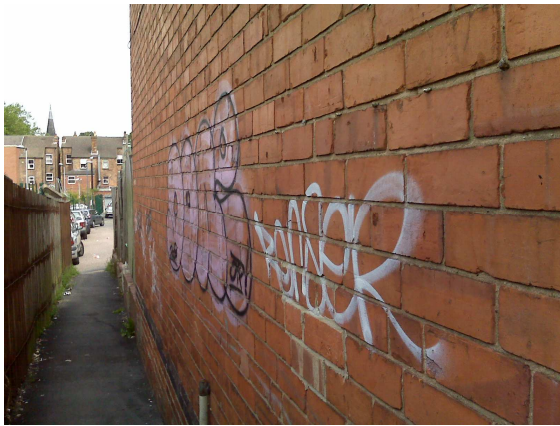
Graffiti on wall of adjacent house
